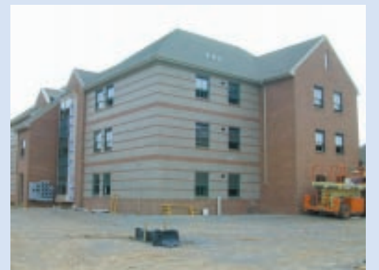
Participants in the Harrisburg campus Alumni Weekend will be among the first to take "hard hat" tours of the new student apartments nearing completion. The housing will replace the Meade Heights community on campus beginning with the January 2002 semester.
